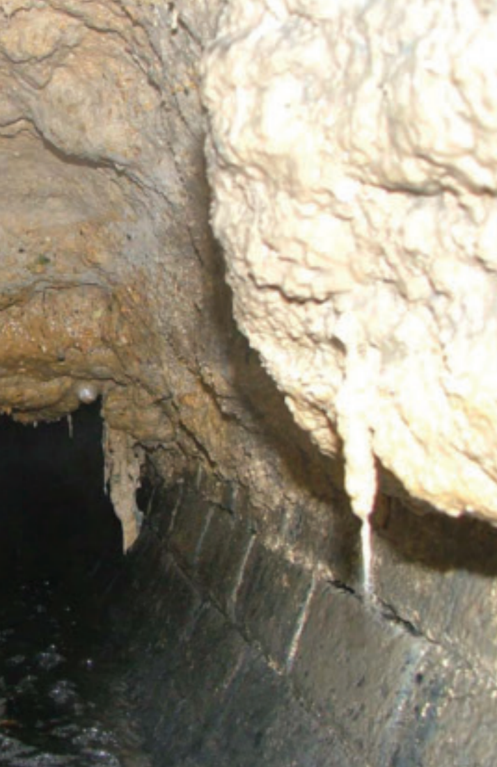
fat oils and grease in a sewer
